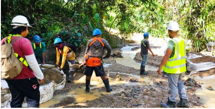
9 TVIRD Environment personnel conduct desilting activities after several days of constant raining.
