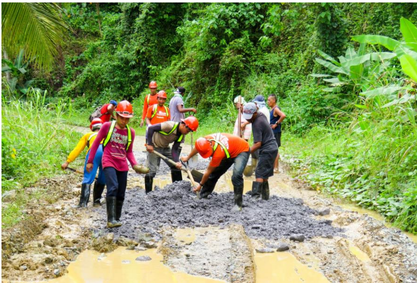
2 Agata and barangay personnel conduct road repairs in Barangay San Vicente in order to mobilize the transportation of relief goods and people.
