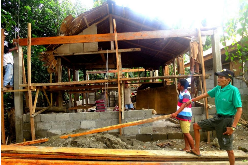
3 Datu Mapaso Moron proudly showcases the ongoing construction of their Tribal Hall – which he personally supervises and which was finally realized through their royalty share.
