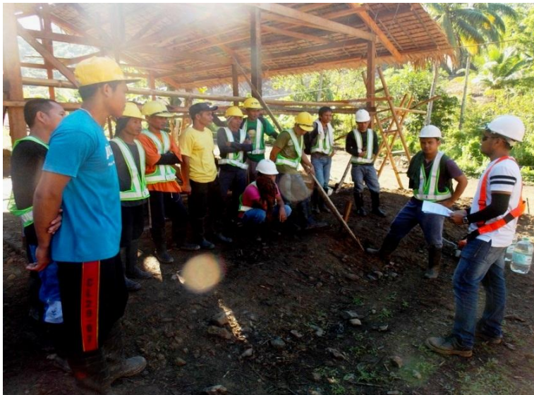
1 AMVI Safety Officer Jake Absin conductes daily safety briefings to field workers on site.
