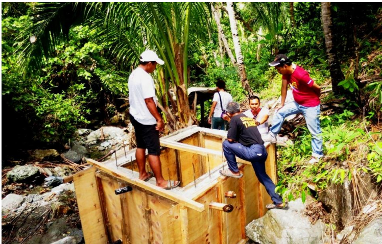
2 Joint inspection. AMVI Personnel and Barangay Lawigan Council Members inspect the progress of their water system.
